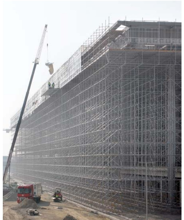
Construction of the new Berlin Brandenburg Airport roof required Layher scaffolding with a surface area of over 530,000 sq ft
