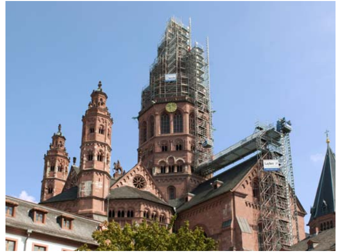
Layher scaffolding and platform stairways on historic cathedral renovation allowed for safer, efficient transfer of goods and workers on the site
